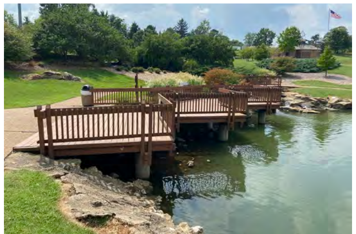
Figure 21: The decks on the south end of the lower pond are used by visitors for fishing and other activities but are deteriorating and require improvement or replacement.
