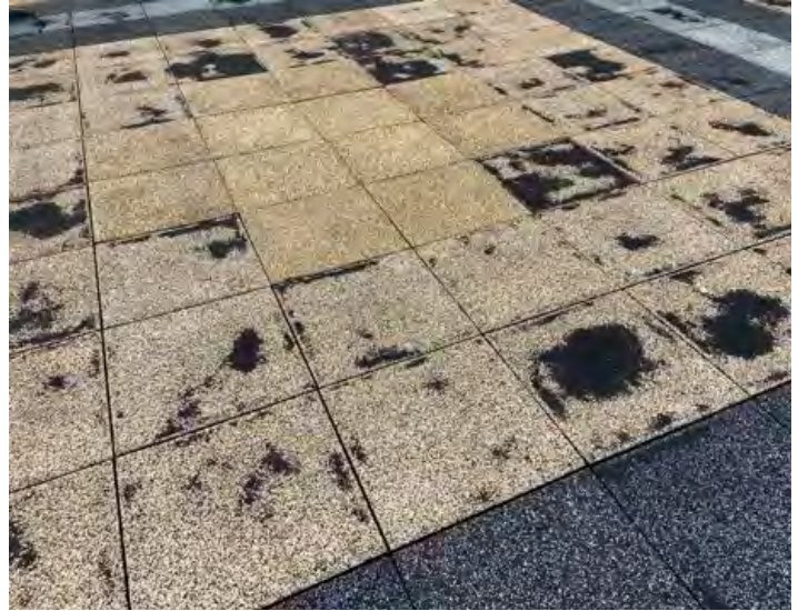
Figure 18: Safety surface tiles are in disrepair and require replacement.
