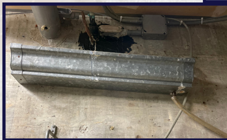
A makeshift gutter has been built to prevent leaks
